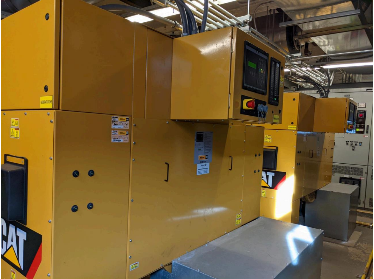
Exhibit 2.10 Interior view – emergency generators at Our Lady of Fatima Medical Center
