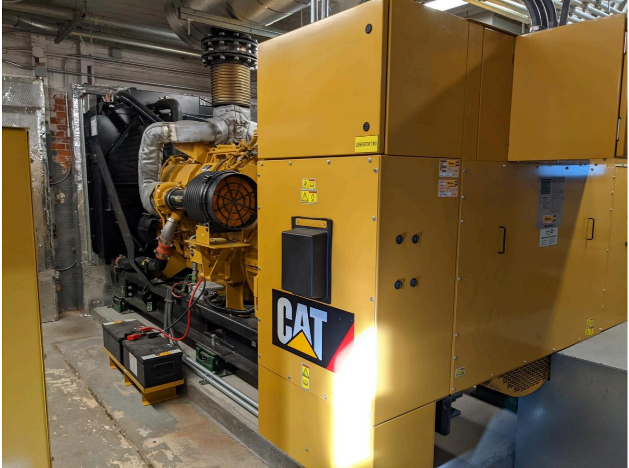
Exhibit 2.9 Interior view – emergency generators at Our Lady of Fatima Medical Center
